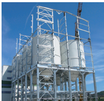
Sand Drying and Transportation, Provodín, Czech Republic Design office: CAB minerals s.r.o., Brno, Czech Republic
